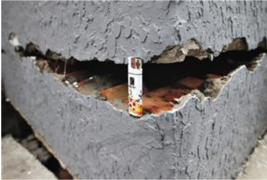
Figure 2. Wall cracks and abscission.
