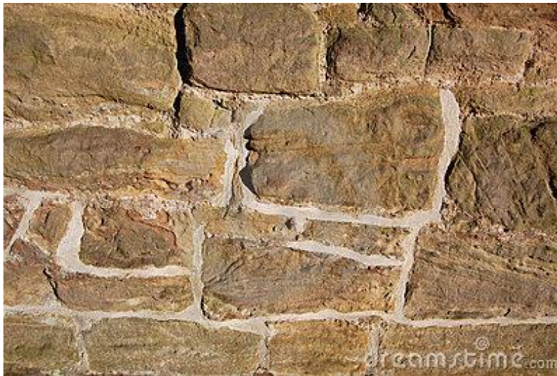
Figure 1. Mismatched color between repointed and original marl.
