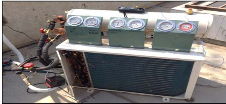
Figure 5. Air cooled condenser with pressure gauges
