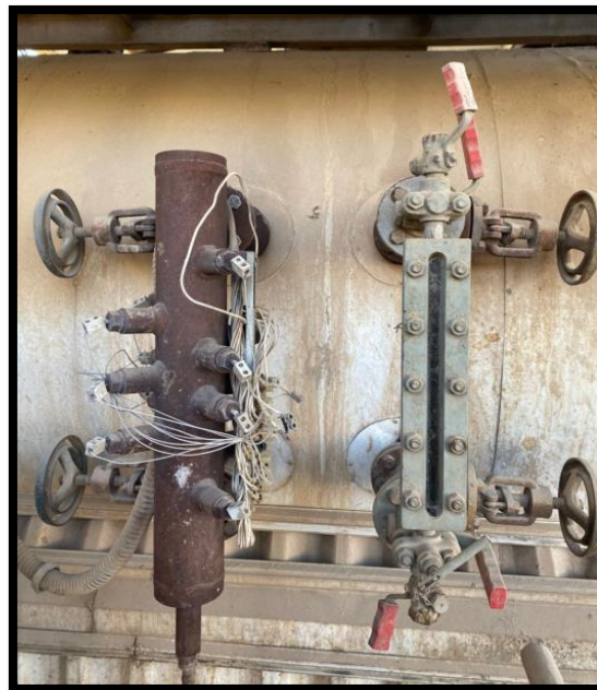
Figure 5. The water level gage in the (Al-Quds power plant).
