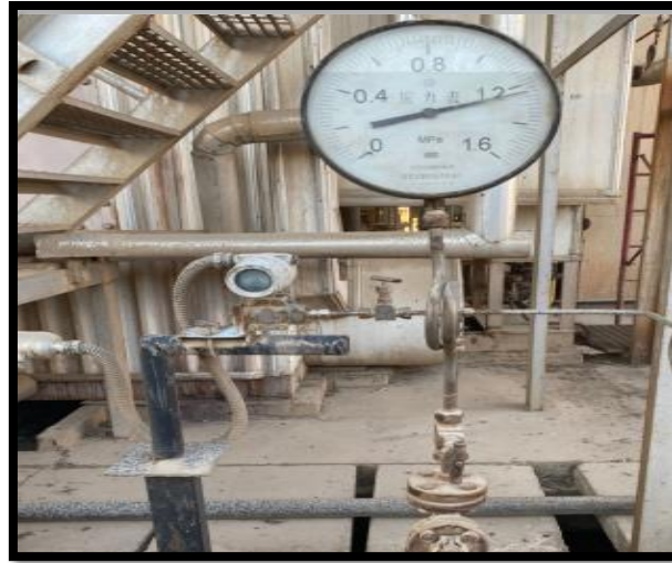
Figure 6. The drum pressure gage in (Al-Quds power plant)
