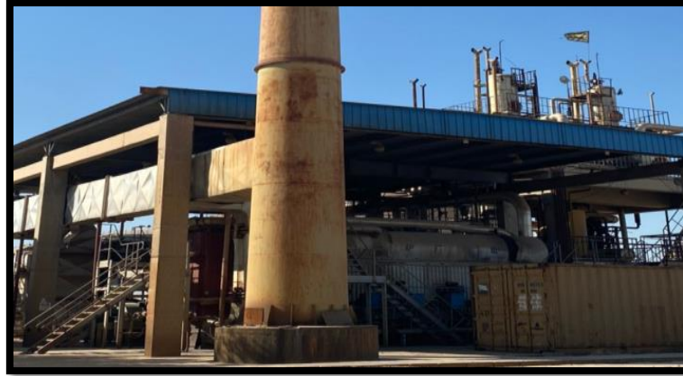
Figure 4. The boiler in (Al-Quds power plant) Baghdad / Iraq
