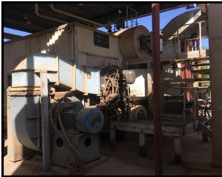
Figure 7. steam generator unit in the (Al-Quds power plant).
